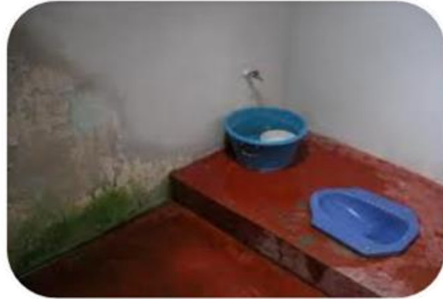
Toilet outside After ExNoRa
