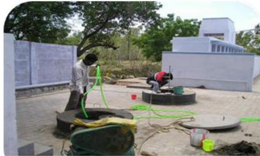
BGS pressure testing preparatory work by Mr.Manickam and Mr.KMS on July 3rd 2005
