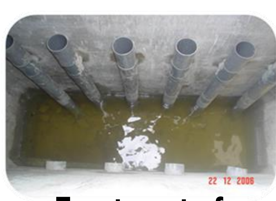
Treatment of Toilet Waste Water
