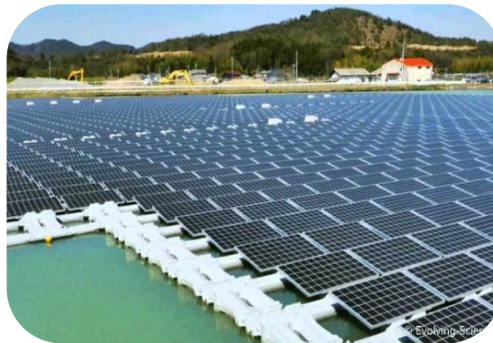
Floating Solar Power Panels
