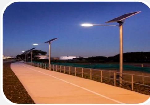
11. Solar Street Lighting
