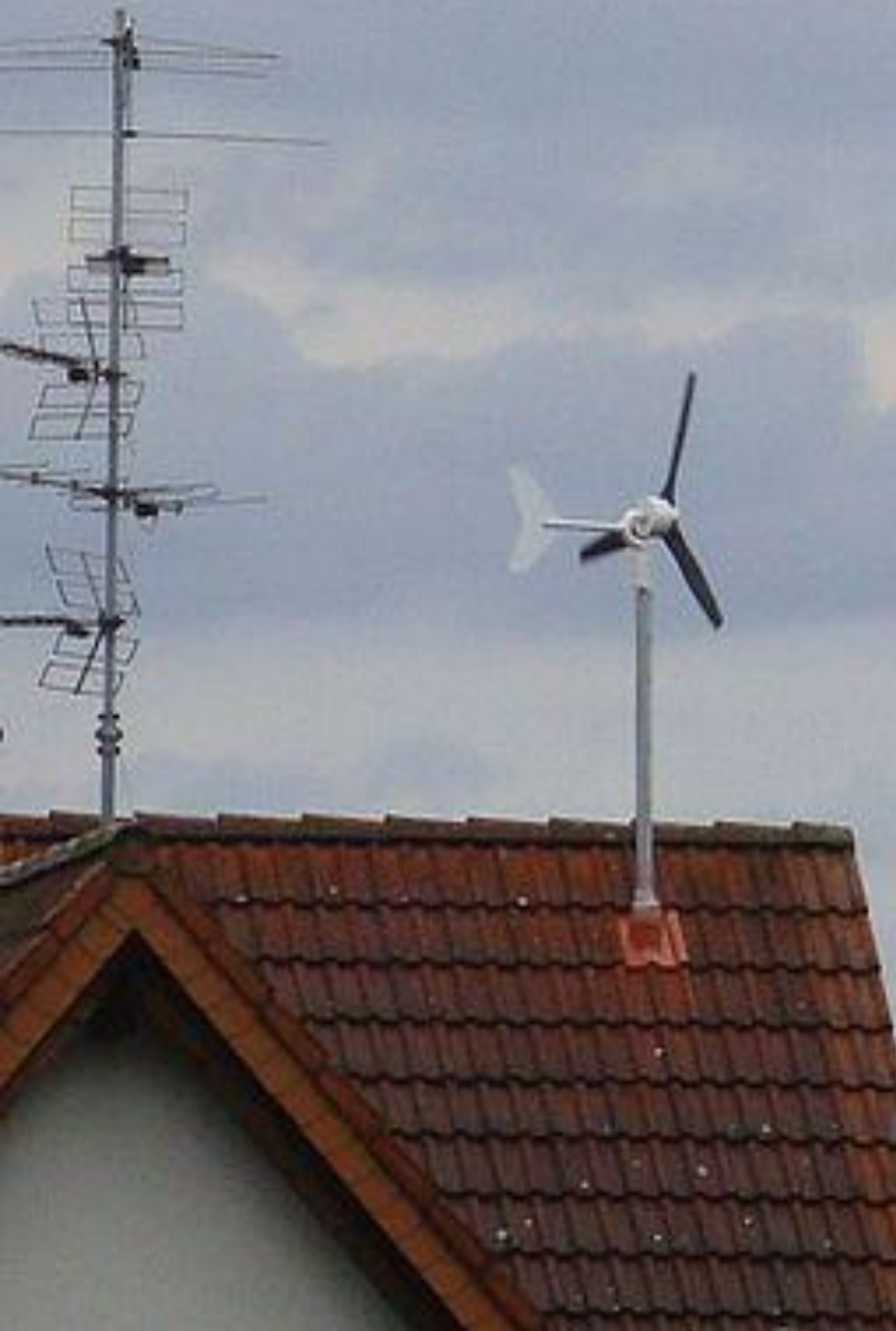
Small wind turbine on roof
