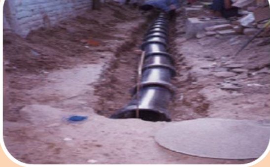
People did Shramdhan and they got a much needed basic amenity so easily
