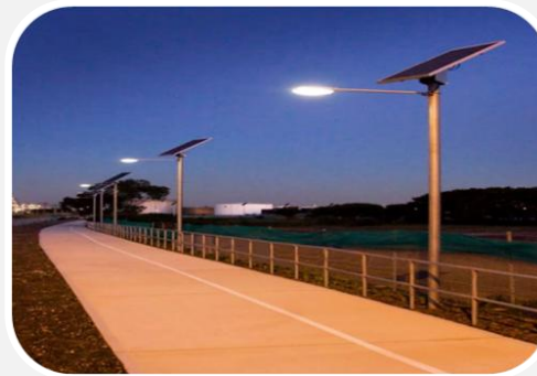
11. Solar Street Lighting
