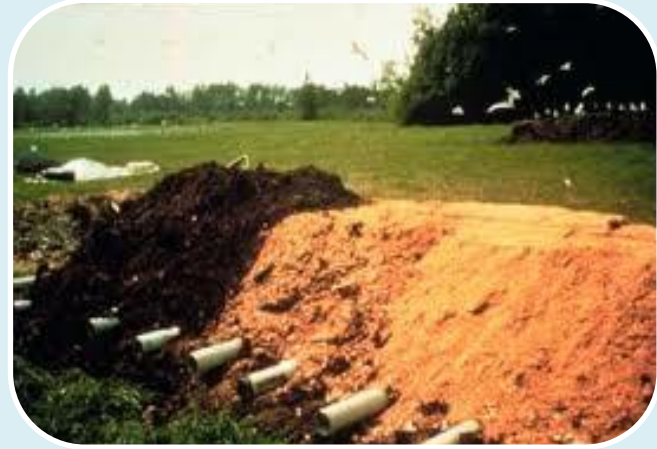
Aerated Pile Composting
