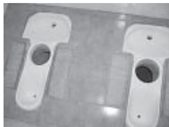
Squatting pans inside the ECOSAN compost toilets at Musiri
